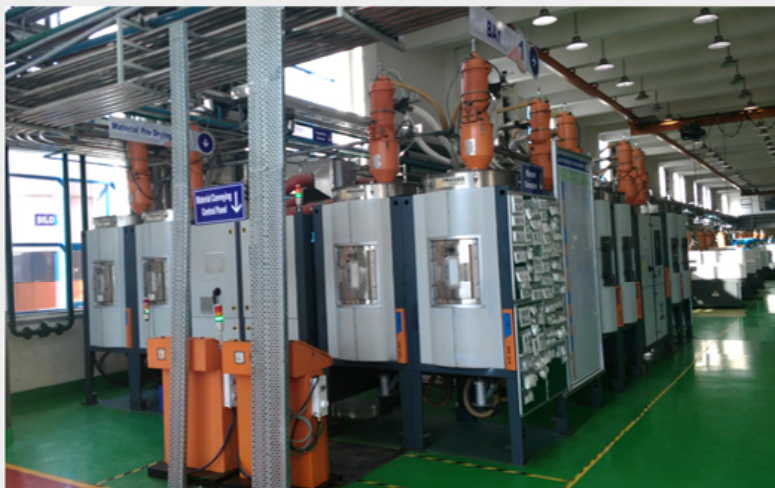
Central Dehumidified Air Dryer with multiple bins
