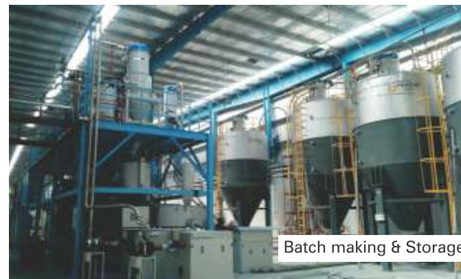
Resin & Filler Unloading
